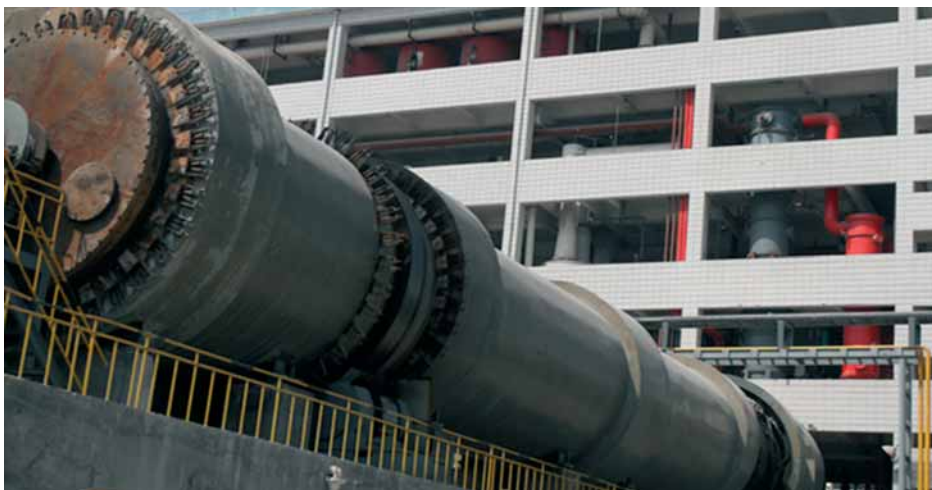
DFD's AlF 3 plant showing the HF kiln in the foreground and HF distillation plant in background
