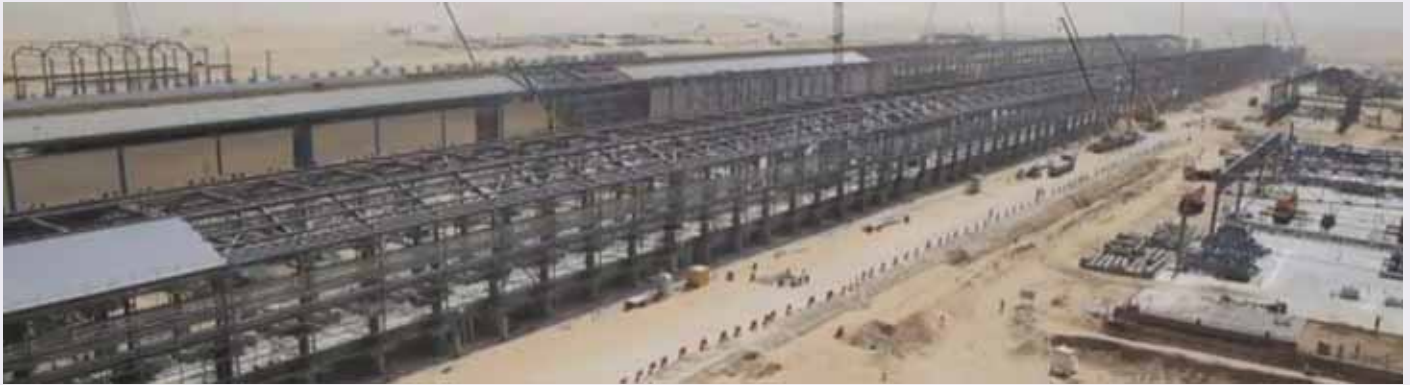
Fig 3 The pot room at the Ma'aden site, Saudi Arabia Pic Source Ma'aden
